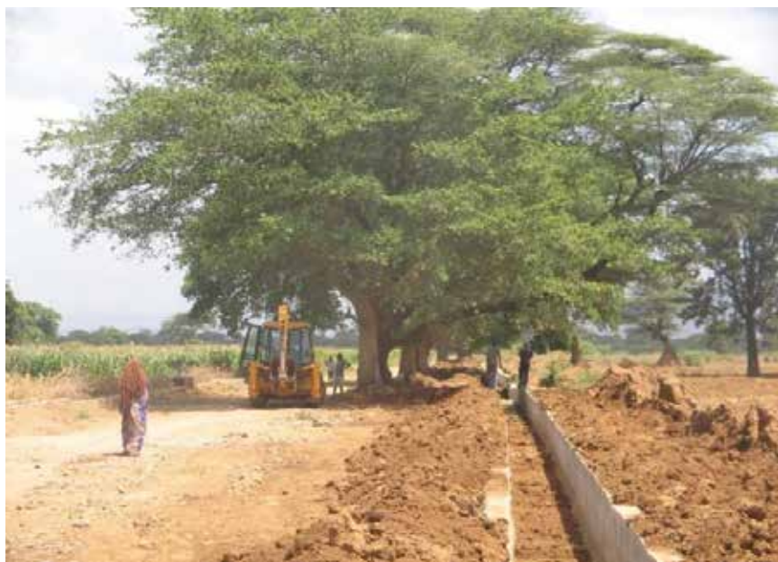
Plate 5: Construction of roads and laying of water pipes in an irrigation site
